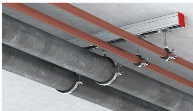
Reconfigurable piping supports
